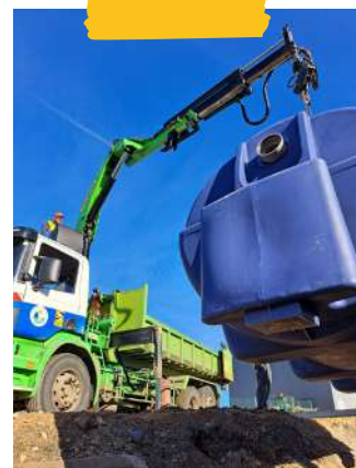
Services techniques CCLPA
